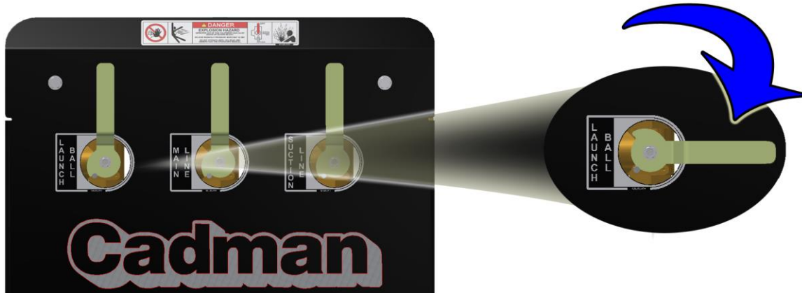
Figure 9 – Launch Ball Valve – Turn to VENT Position
